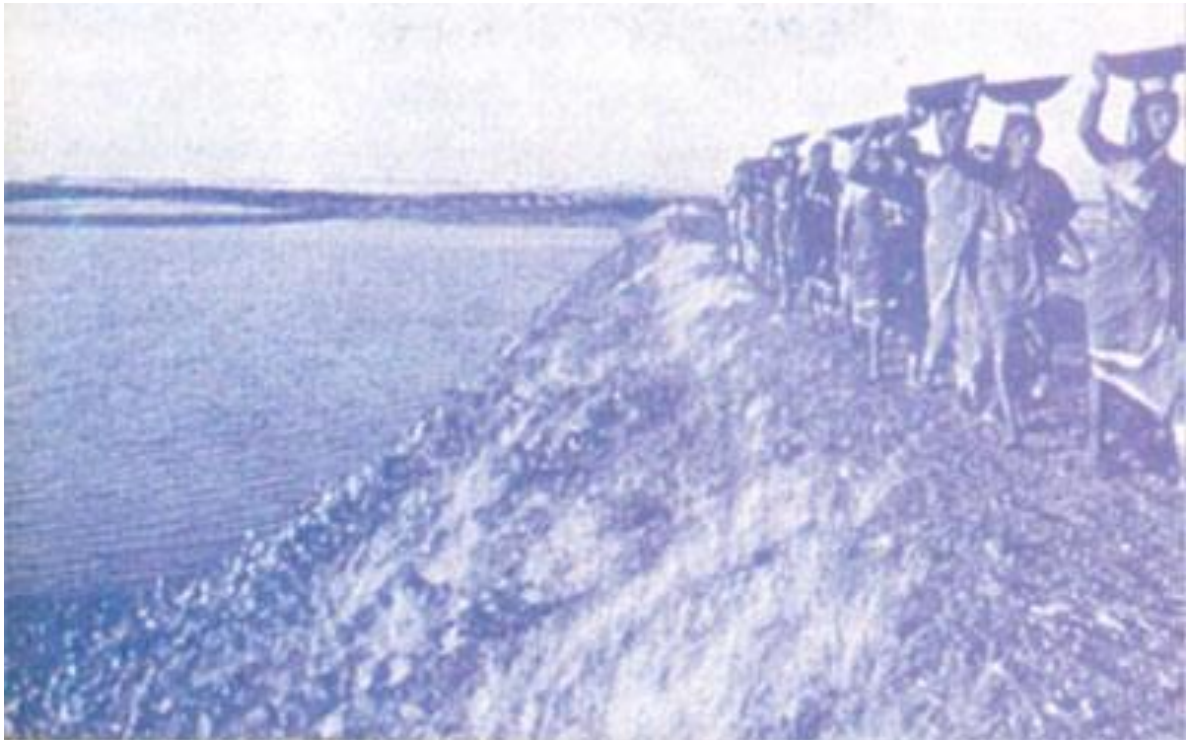
Photo 1.1 Percolation tank construction near Baramati, Maharashtra, India, in the 1970s with women carrying murum and clay one bowl at a time to patiently construct the designed embankment. ( Photo from Agricultural Trust Baramati ).
