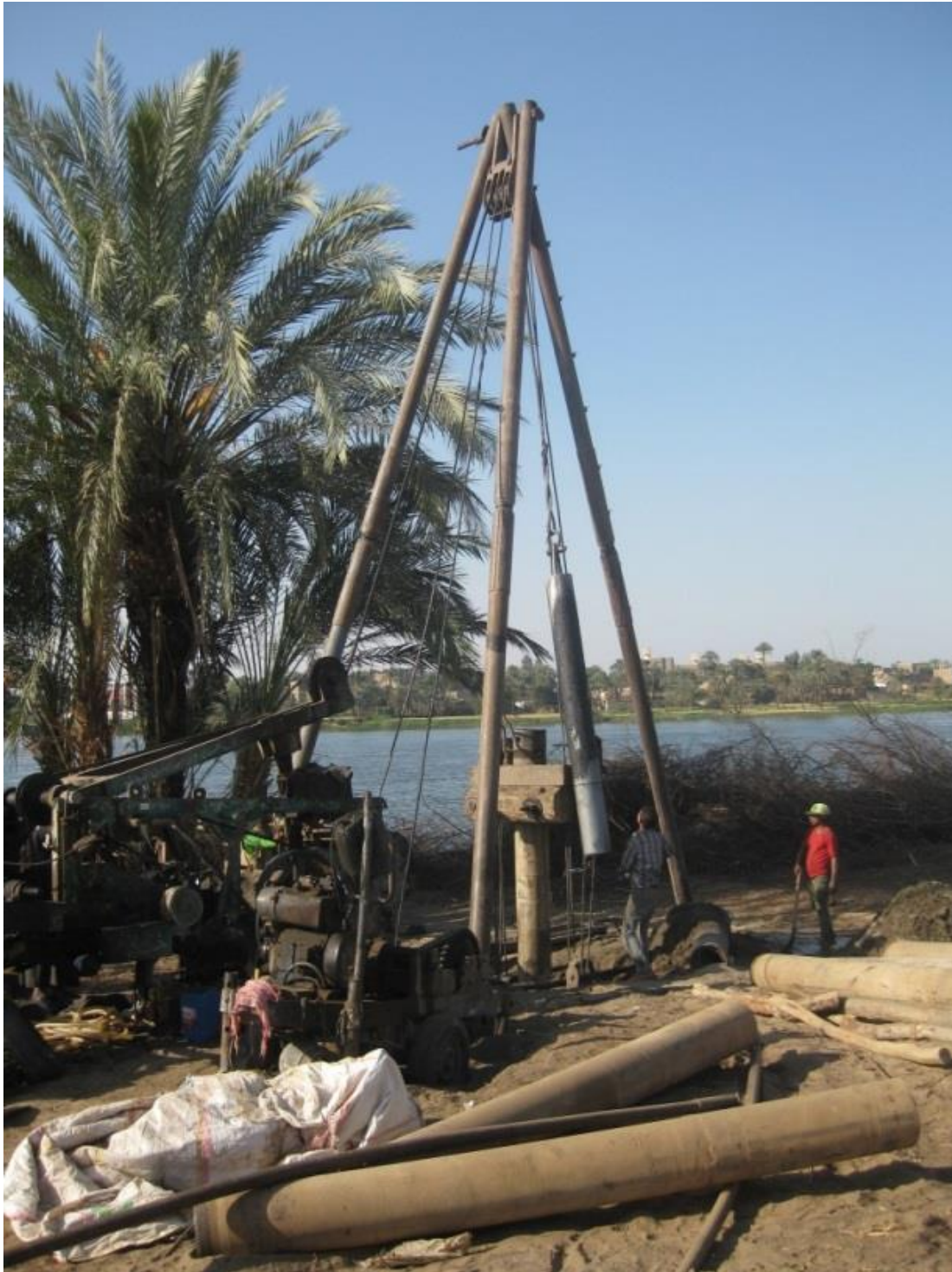
Drilling of river bank filtration wells at the River Nile, Luxor, Egypt, March 2018. Seasonal low river water level, frequent spills of oil and other pollutants and high turbidity during high flow cause problems in surface water abstraction and subsequent treatment. A short distance between the abstraction wells and the river bank is sufficient to remove particles, to buffer spills and to ensure a high portion of bank filtrate and a low portion of manganese-rich land-side groundwater. (Photograph courtesy of T. Grischek, HTWD)
